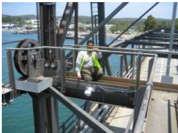
Figure 12: Sensor deployment – Bateman’s Bay Bridge
